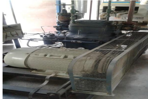
Figure 5: Chiller Compressor in Jorethang Plant
